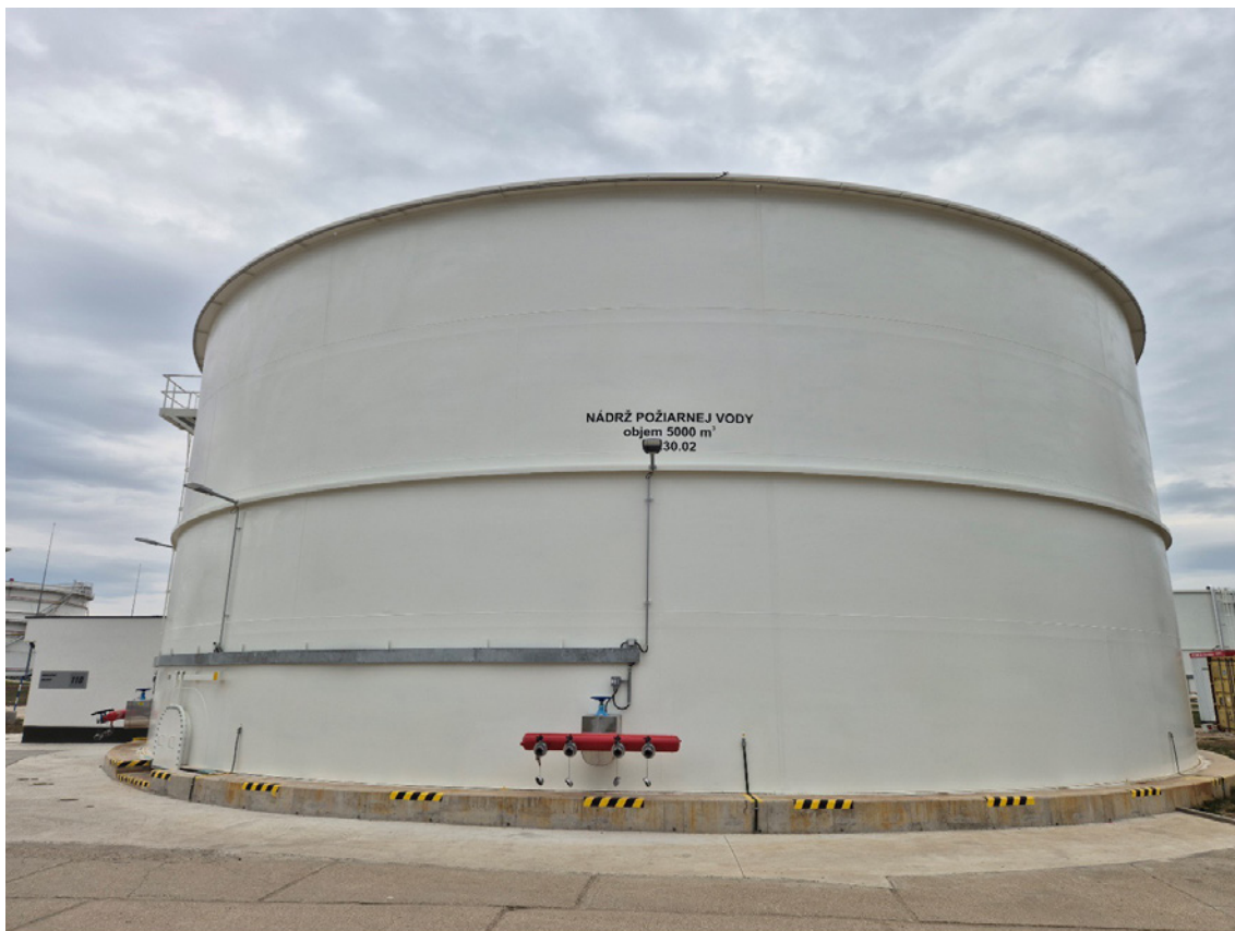
Fig.: New 5 000 m 3 fire water tank at PS 4 Tupá.
