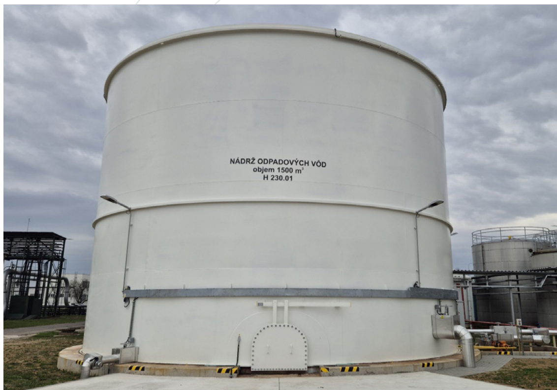
Fig. 1: New 1 500 m 3 wastewater tank at PS 4 Tupá.
